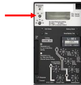
Figure 6. Integral Maintenance Switch
