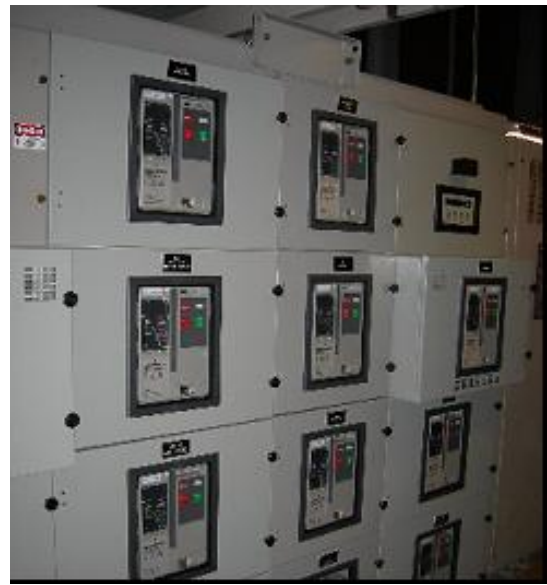
Figure 5. Retrofilled Fuses with Breakers Example
