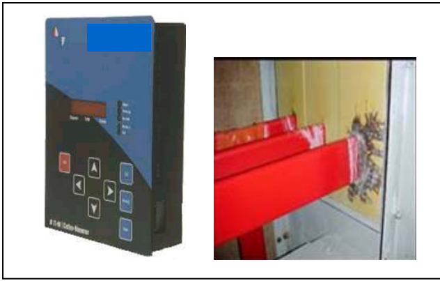
Figure 18. Partial Discharge Relay and Switchgear with Pending Failure
