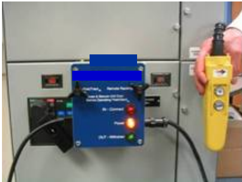
Figure 11. New LV Motor Control Center with Remote Racking Device
